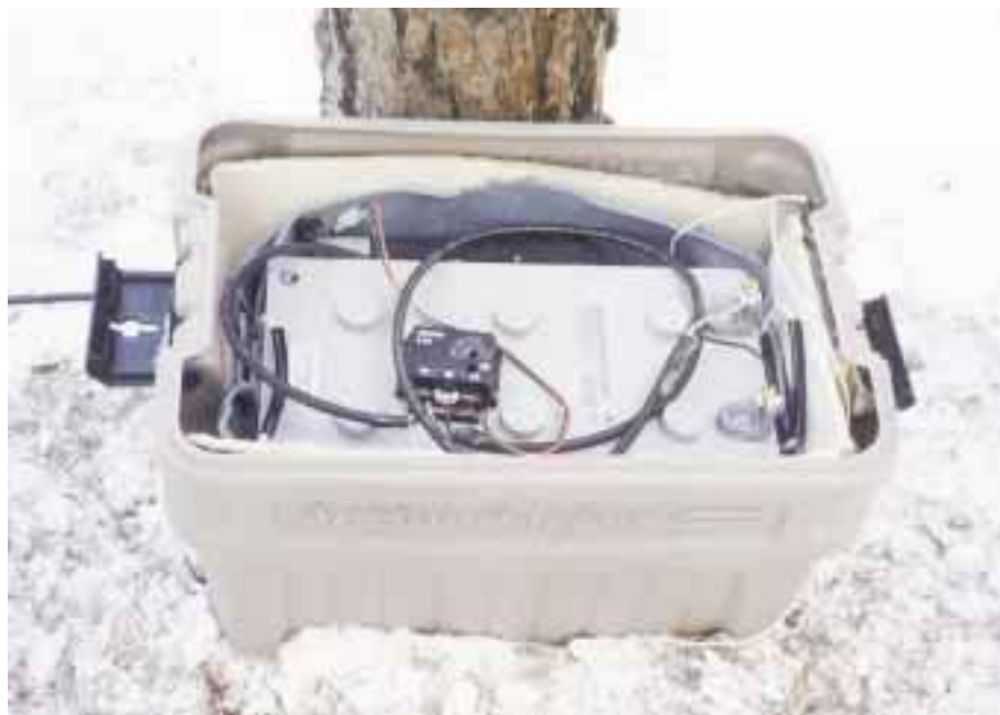
A plastic tub protects the 280 amp-hour Deka gel-cell battery, Solsum 5 amp charge controller, and Telemobile Ptel radiotelephone.
